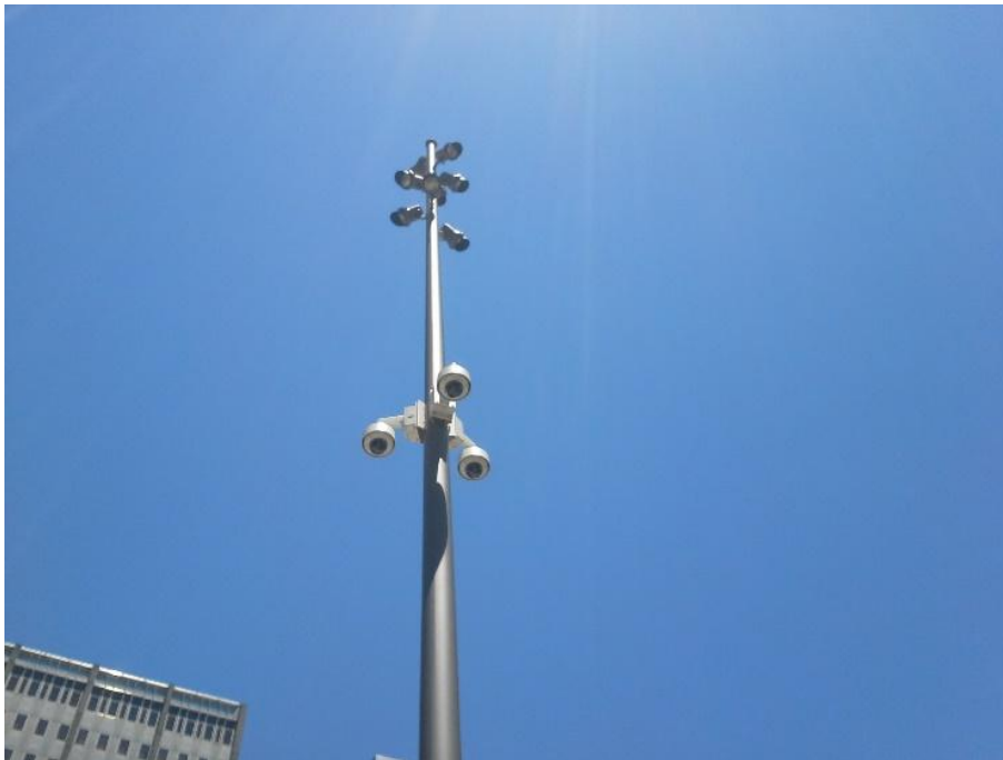
Figure 4: Security cameras, Philadelphia, PA. (Photo by author.)
